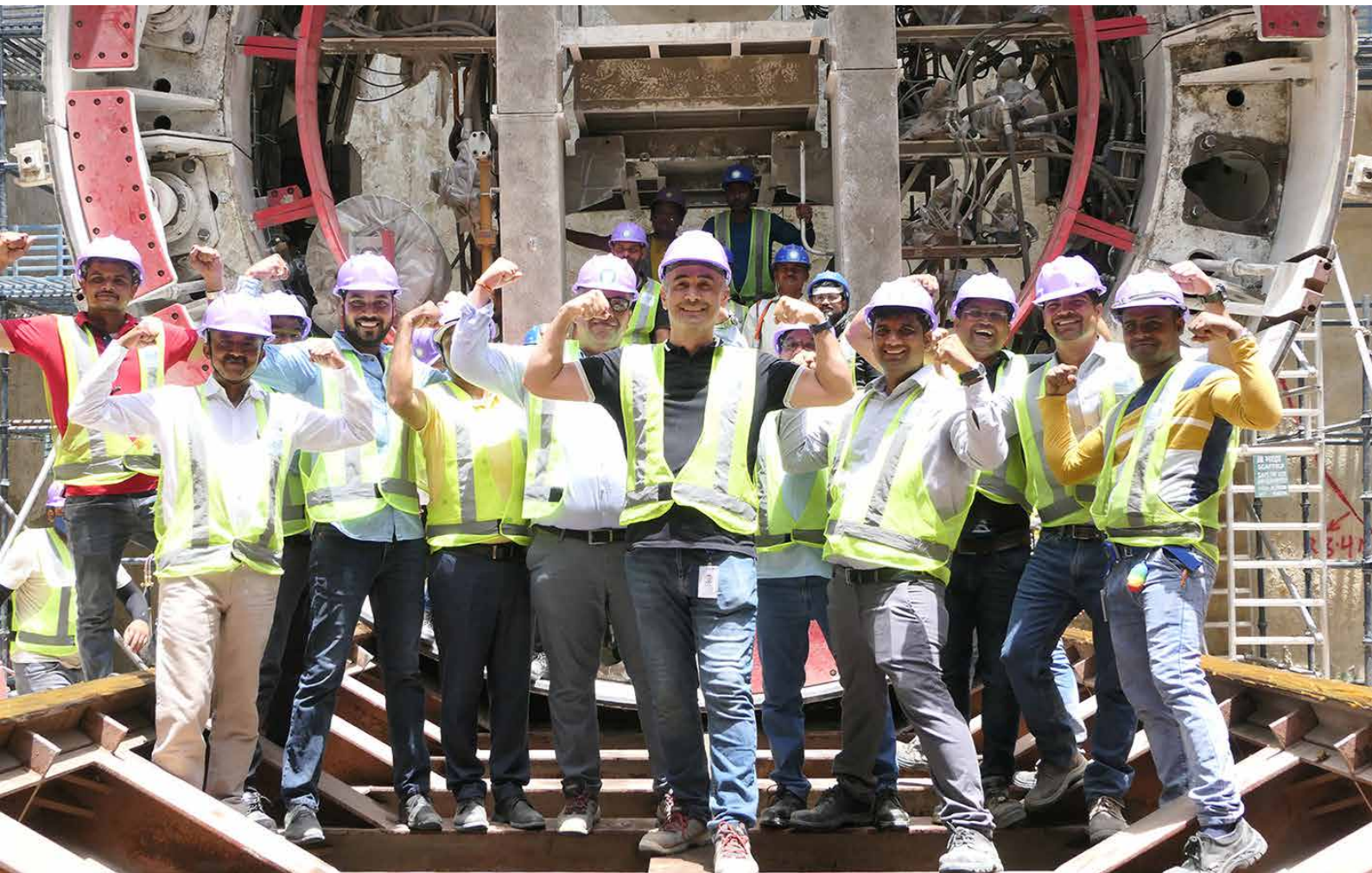
Gulermak/Sam India JV gets ready to commence tunnelling on the Corridor-1 of Kanpur MRTS Project in India.
