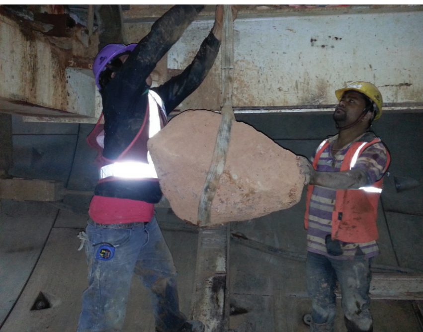
Project CC-07: Boulders of sizes over 600mm were found passing through the TBM Screw Conveyor
